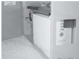
Battery System Status Indicators
