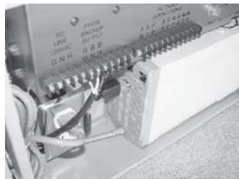
All Connections to APC Backup are Modular
